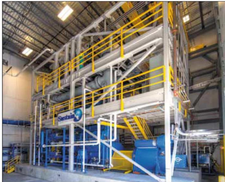
Figure 70 SustainX's 1,5MW isothermal CAES in Seabrook, New Hampshire, USA
