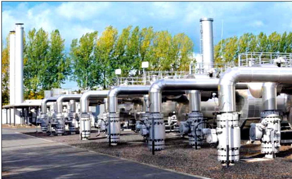
Figure 66 Surface equipment at the Epe salt cavern facility in Germany
