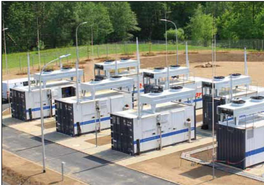
Figure 71 The E.ON & Swissgas 2MW power-to-gas unit in Falkenhagen (Germany)
